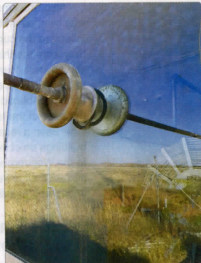
Photo 3: The feeder exiting the transmitter hut.
