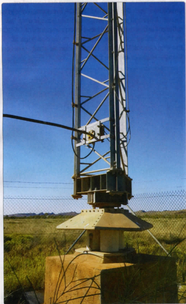
Photo 4: The Woodbrook antenna base and feed arrangement.
