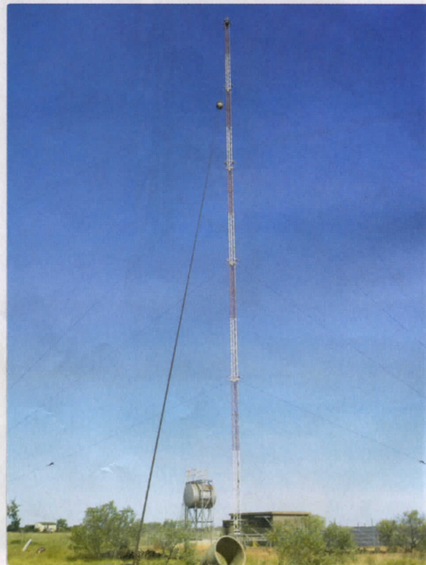
Photo 8: The antenna at the De Grey site.
